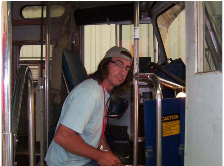
Anthony Carideo shown installing a new headlight resistor in PCC #532 on Track #3 in our A Shop. Dave Slater Photo
