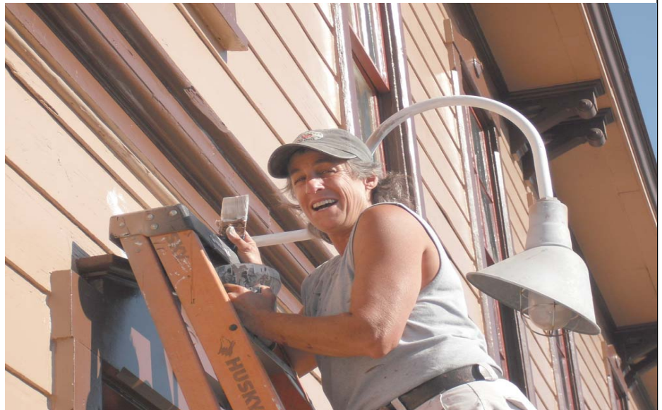
Lori Kaye does last minute touch-ups on the Depot after its major exterior paint work. Photo by Jeff Trimble
